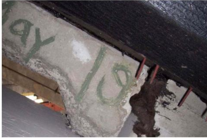
Figure 7. Broken Concrete in Roof [6]
