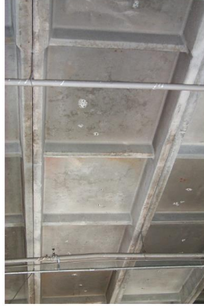
Figure 6. Sprinkler System and Spalling from Roof System [6]
